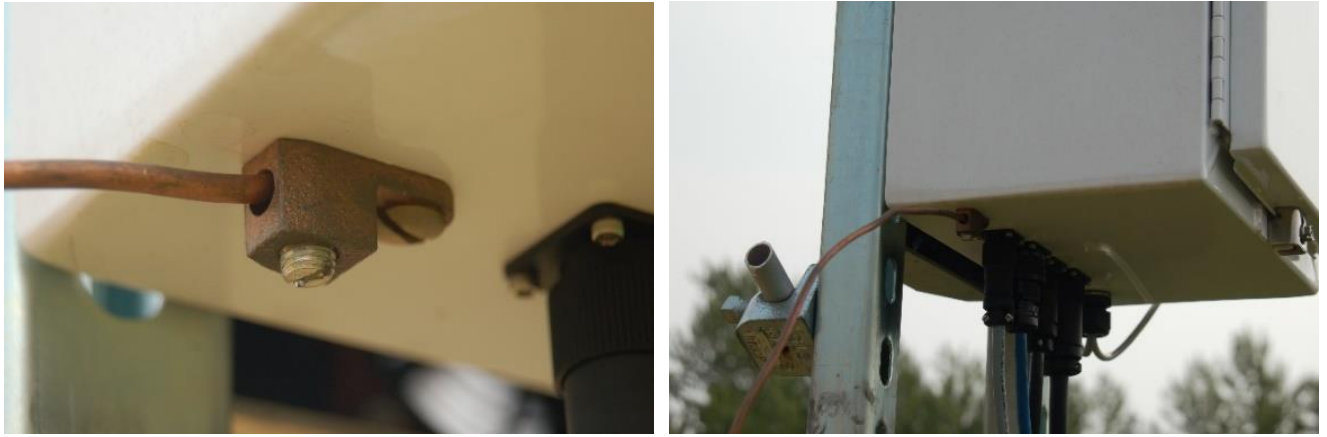
Figure 6. Images of the ground lug on the bottom of the ICI.
